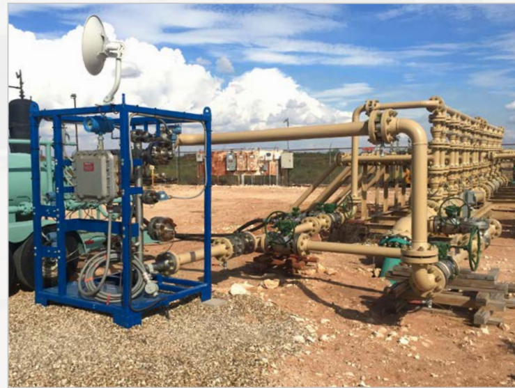
MPFM with radio link to SCADA, Texas, 2012
