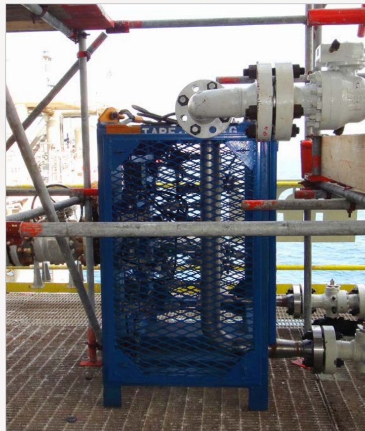
MPFM installation offshore, Qatar, 2011
